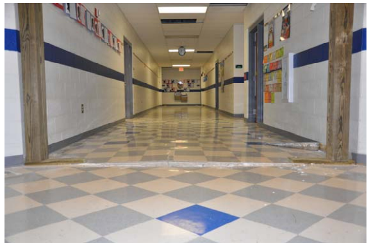
CHANGES IN THE FLOOR SURFACE - BENLD, IL
