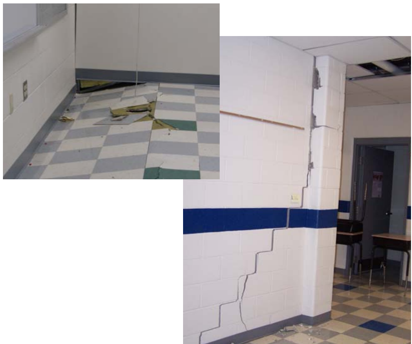
FLOOR AND WALL CRACKING - BENLD, IL
